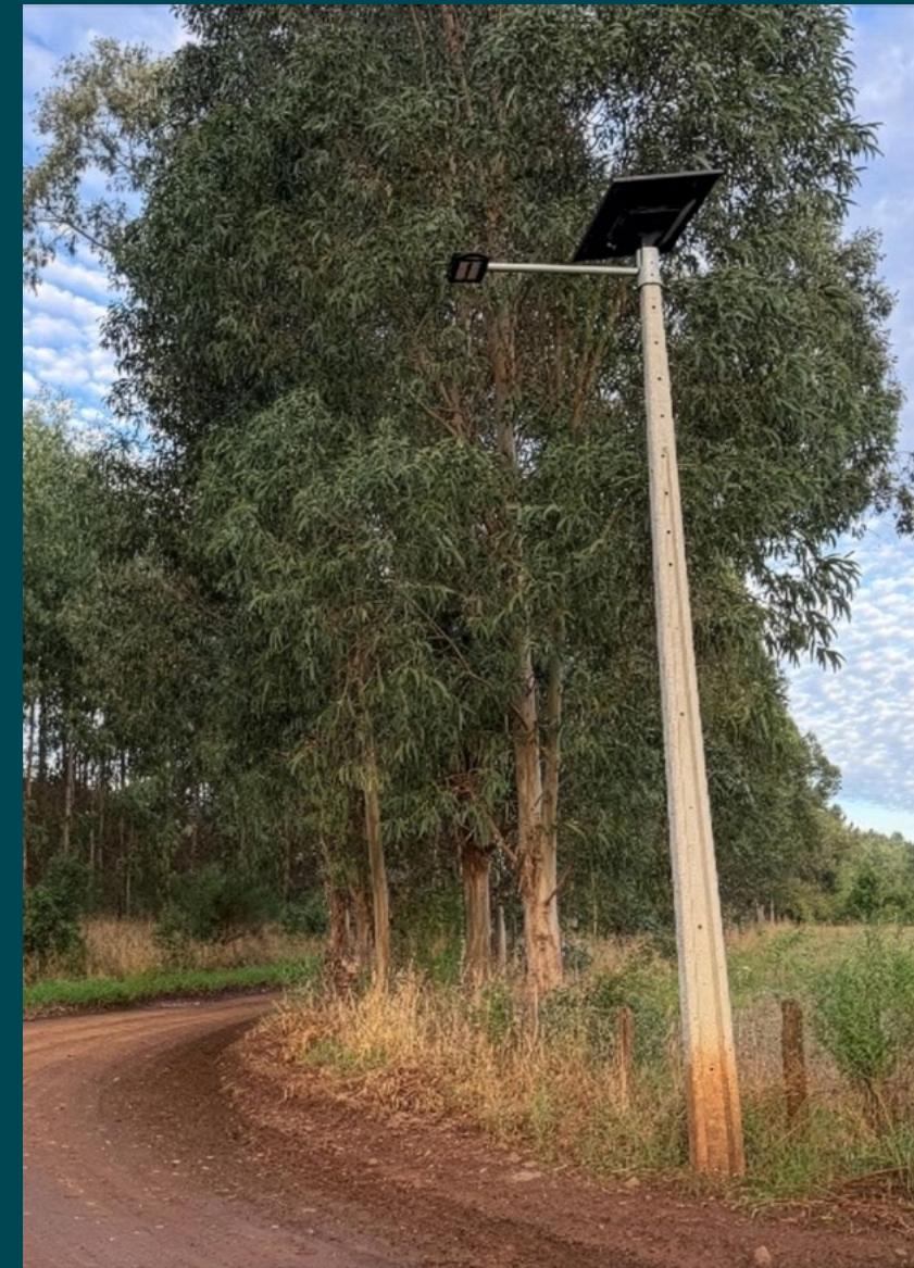
Solar-powered street lighting. Source: Nala Renewables
