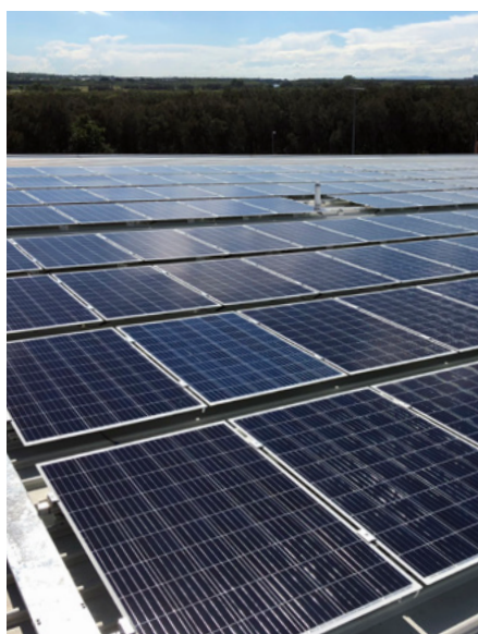
Solar panels mounted on the roof of one of the airport's car parks
