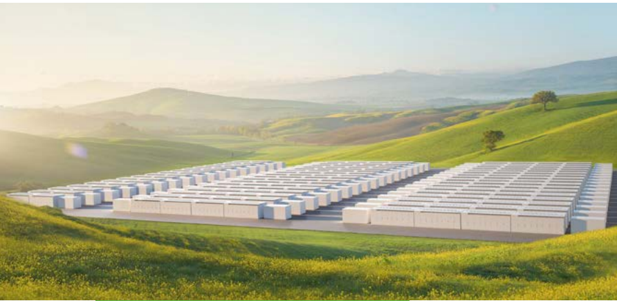
Battery storage is a relatively new technology that is helping decarbonise the electric grid.
